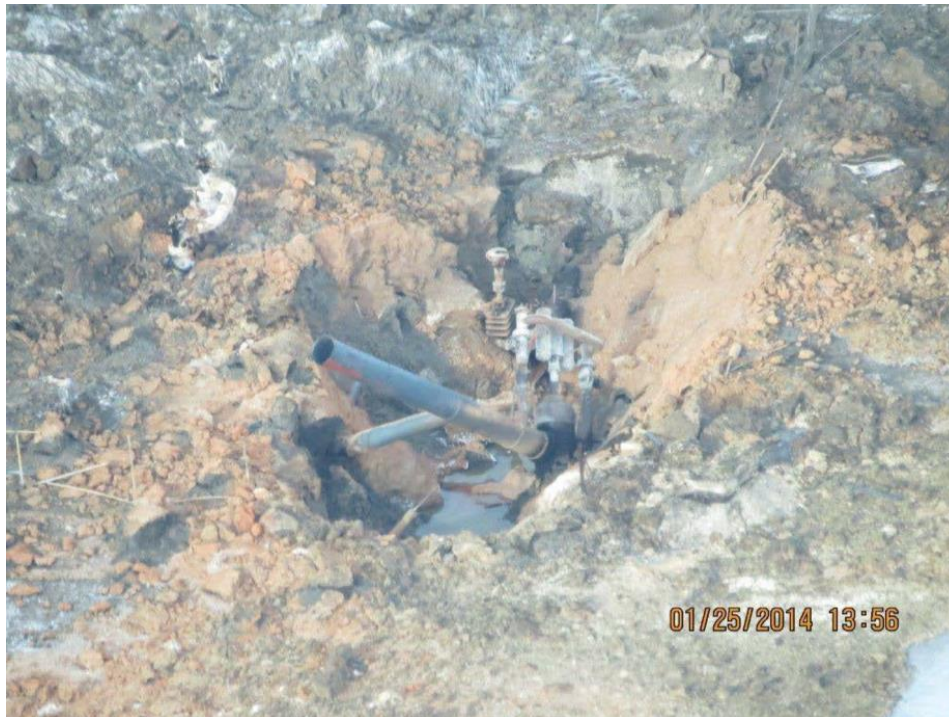
Figure 2.1: Uplift of the valve and pipeline section following rupture and explosion. Photo credit: courtesy of Transportation Safety Board of Canada (2014).
