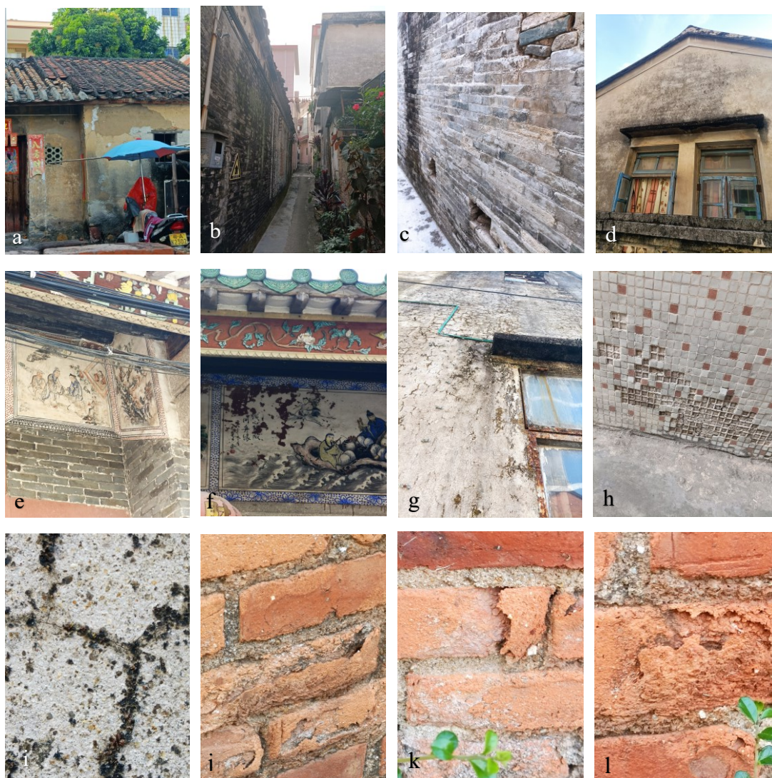
Fig. 1-2 Appearance of the exterior wall of a traditional village dwelling in Nansha, Guangzhou affected by salt erosion
