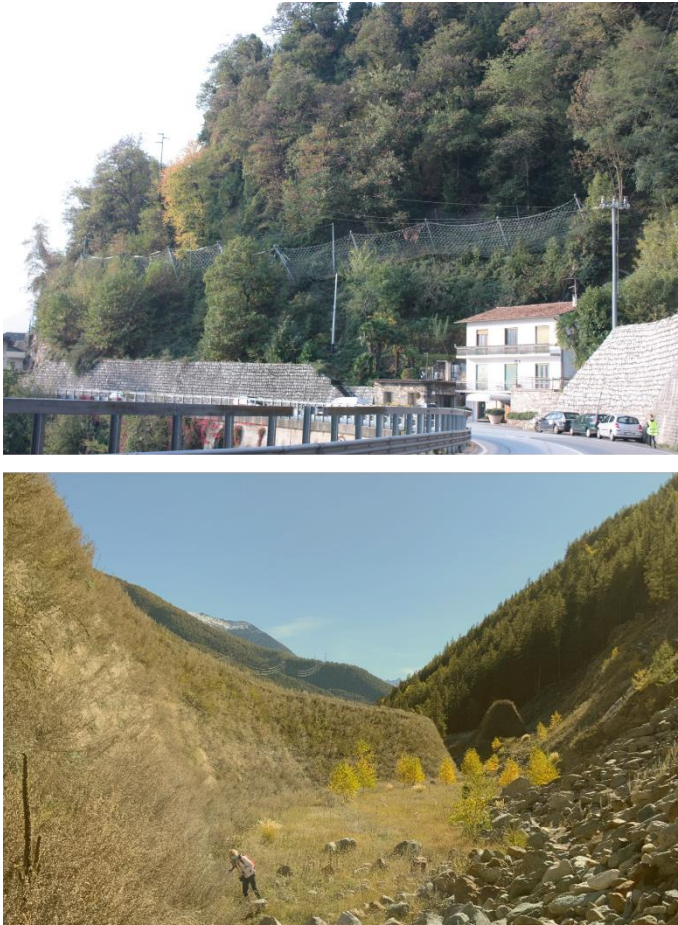
Figure 1. In the top, view of a rockfall net fence along a road. In the bottom, view of a rockfall earth embankment.
