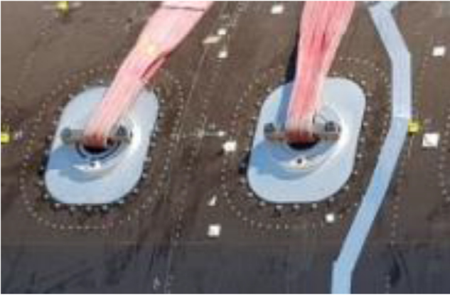
Fig. 2. A) Bands used to raise the section fuselage; B) Metal plug with handle.
