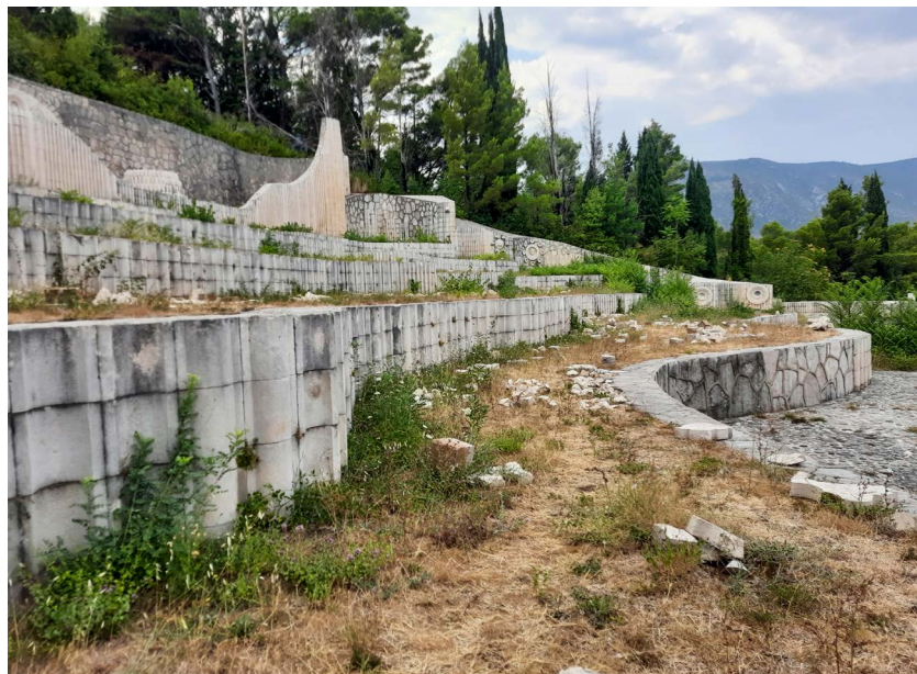
Detail of damaged burial terraces and displaced stone elements, evidencing the material consequences of vandalism and the erosion of the cemetery's funerary function.
