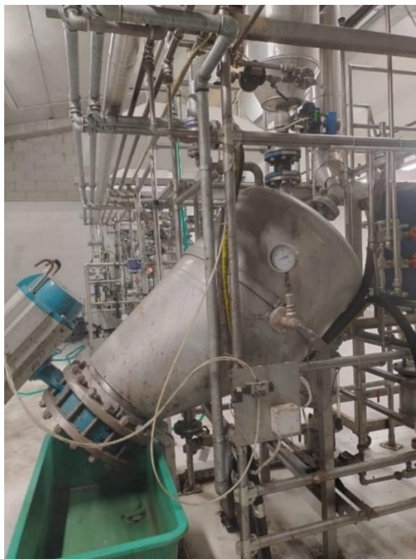
Figure 3.4: Steam explosion expansion vessel
