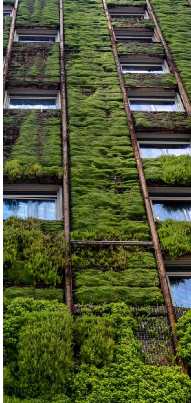
Figure 5. Vertical greenery systems applied to a building facade
