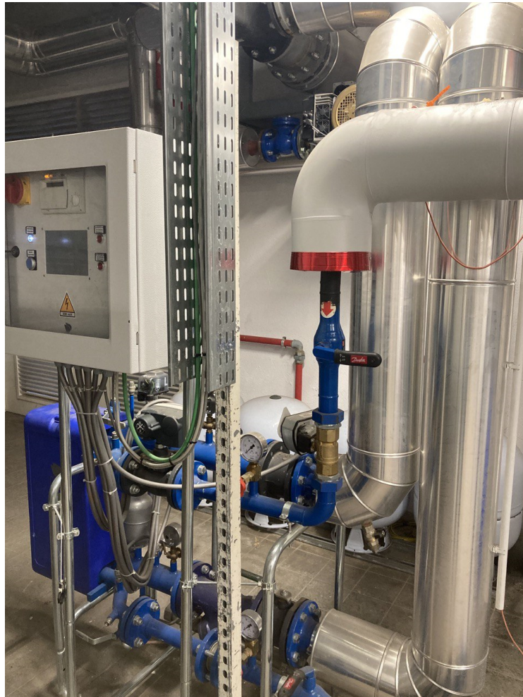
Fig. 3.16 District heating substation (heat source dedicated to the experimental testing rig)
