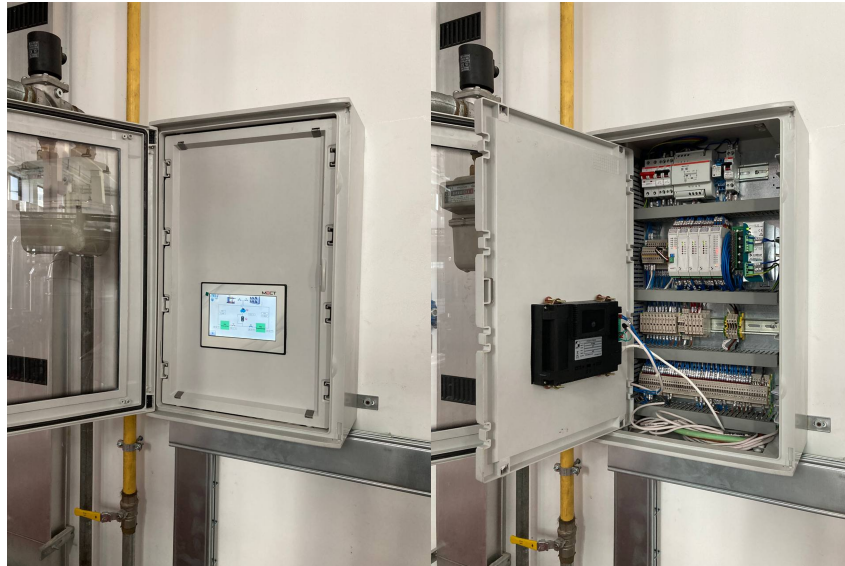
Fig. 3.22 Programmable Logic Controller (PLC) dedicated to the experimental testing rig
