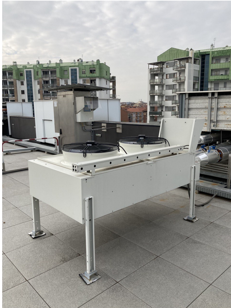
Fig. 3.18 Dry cooler (heat sink dedicated to the experimental testing rig)
