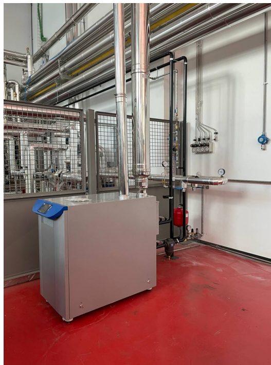
Fig. 6.6 Detail of the micro-CHP installed at the Energy Center pilot site
