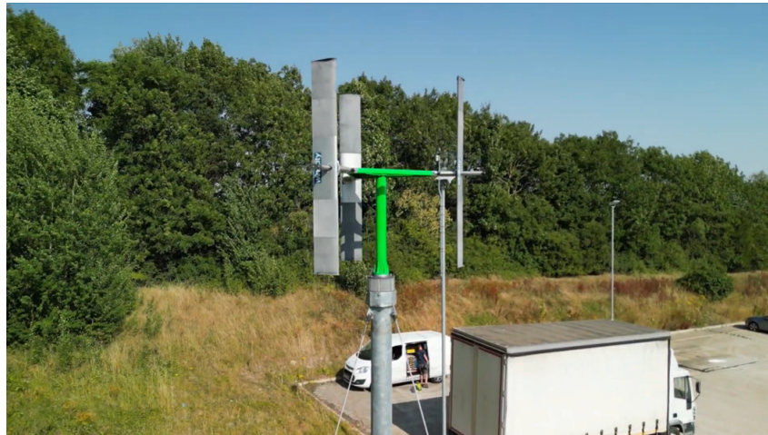
Fig. 6.7 Detail of the Vertical Axis Wind Turbine installed at the Corby pilot site [156]
