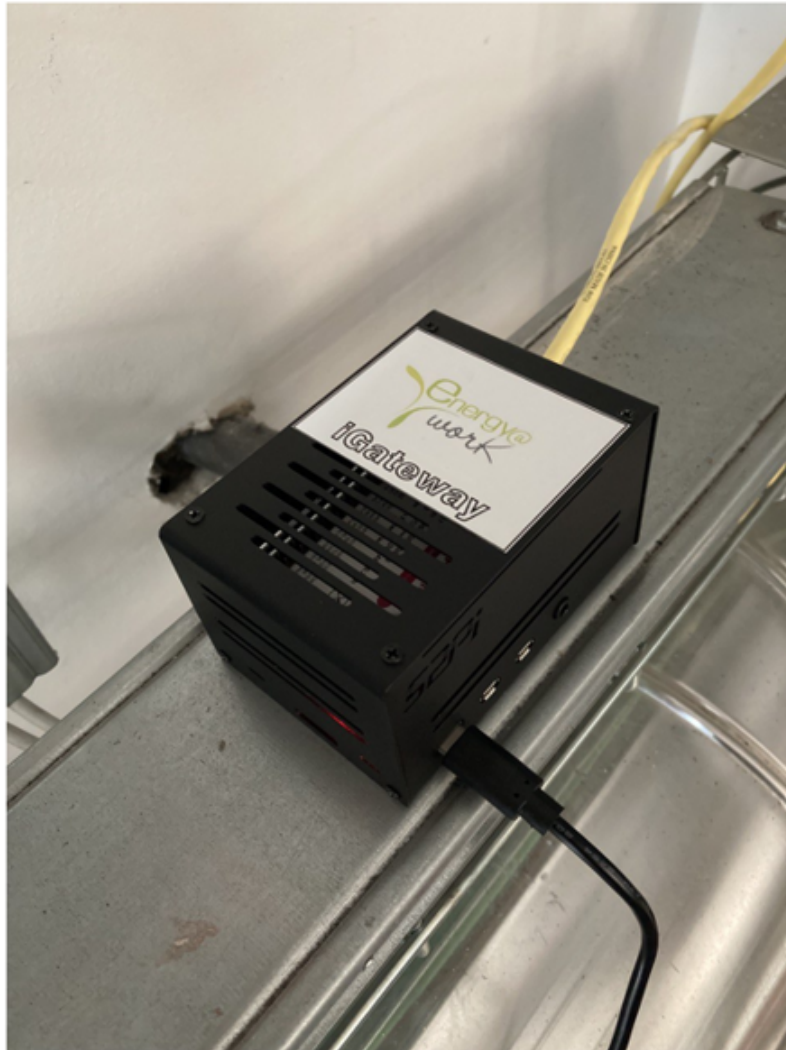
Fig. 6.5 Detail of the i-Gateway installed at the Energy Center pilot site
