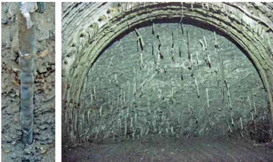
Fig. 10 – PERGround© bar removed after injection (left). Tunnel face improved by means of PERGround© (right).
