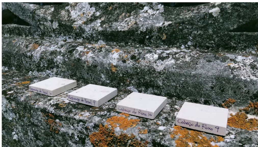
Fig. 2. Uncoated and SiO x deposited stone samples placed on the roof of Batalha Monastery (from left to right, 1st and 3rd covered with SiO x thin film, 2nd and 4th uncoated).
