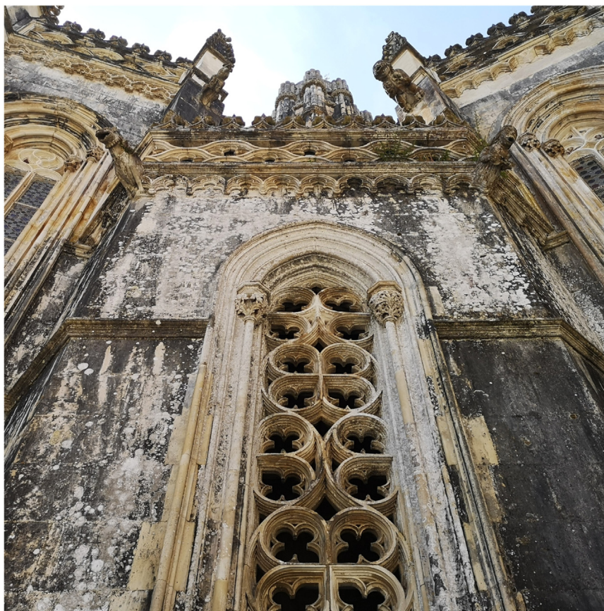
Fig. 1. Batalha Monastery, Portugal. Limestone heavily affected by microbial deterioration and lichenous patinas.
