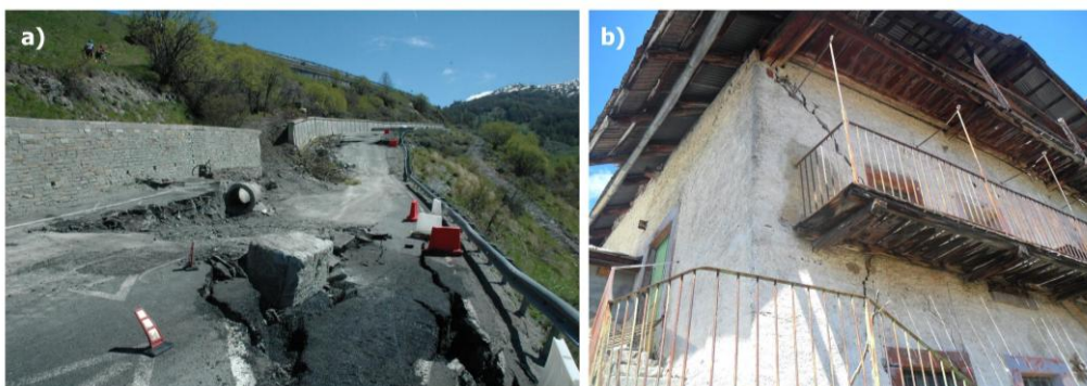
Figure 1.2 Main impact of the evolution of the DsGSD on anthropic element recognised in the Italian Western Alps: the Champlas du Col landslide with (a) significant damage to roads (SP23R) due to secondary landslides associated with the DsGSD and (b) injuries to buildings.
