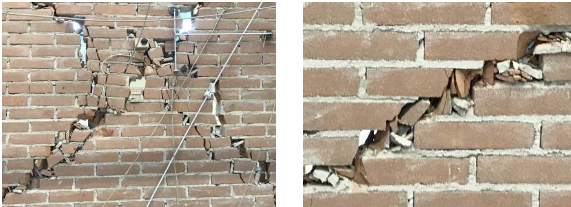
Figure: Highly brittle and discontinuous phenomena observed in masonry failure
