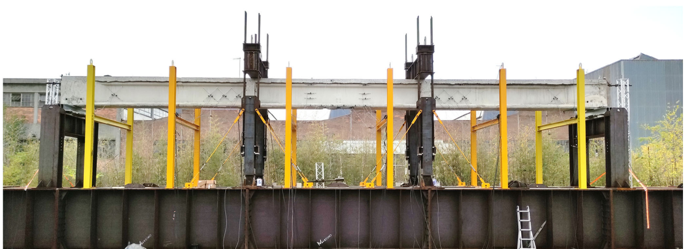
FIGURE 5 Steel reaction frame with a deck beam in a four-point bending test configuration.
