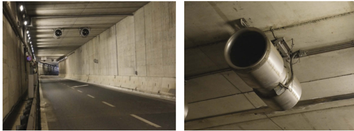
Figure 3. Jet fans positioned in pairs on the roof of a one-way road tunnel (left) and a detailed view of a single jet fan (right).
