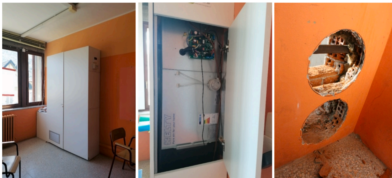
Fig. 1. (a) one of the installed DMV units; (b) the system controlling board; (c) a moment of the installation.
