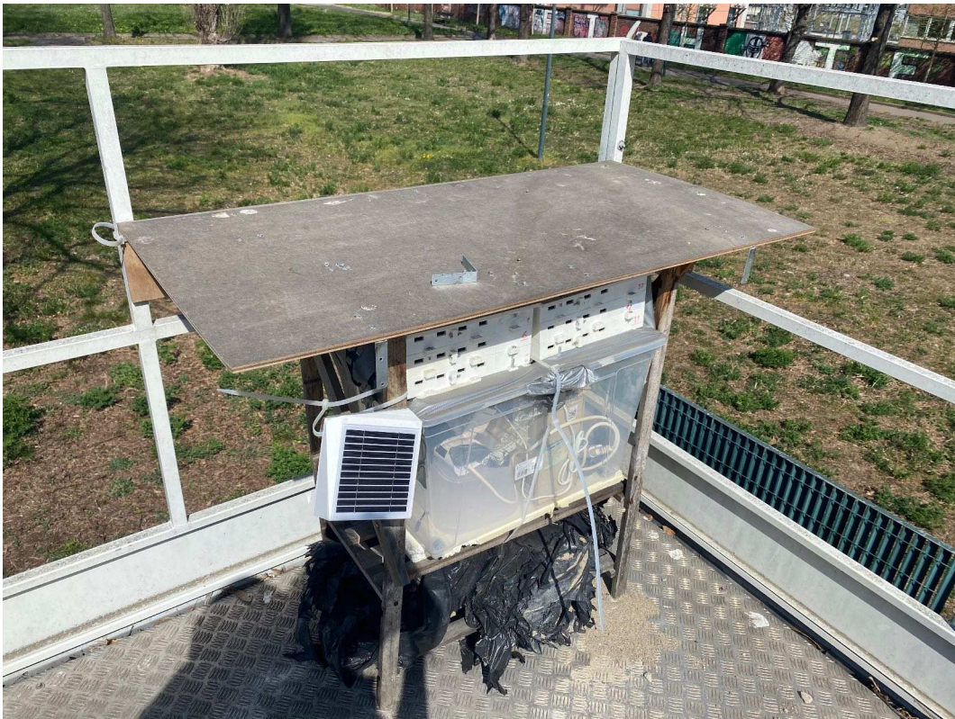
Fig. 5.3 Setup of Air Monitoring Stations on the Rooftop of the Rubino Station
