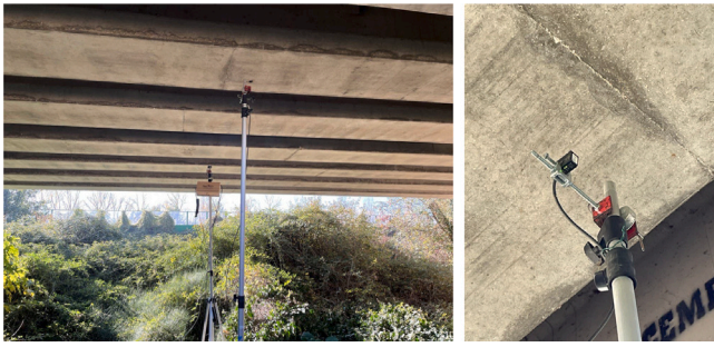
Fig. 12. View of the sensors layout and experimental setup in the Orte-Falconara bridge (1st case study) for the bridge deflection measurement using laser sensors under the train transit.
