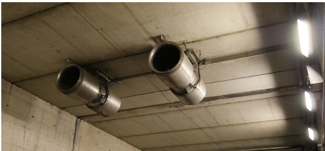
Figure 2. Example of a pair of jet fans anchored to the tunnel roof, used in the longitudinal ventilation of a one-way road tunnel, with airflow in the same direction as the vehicular flow.
