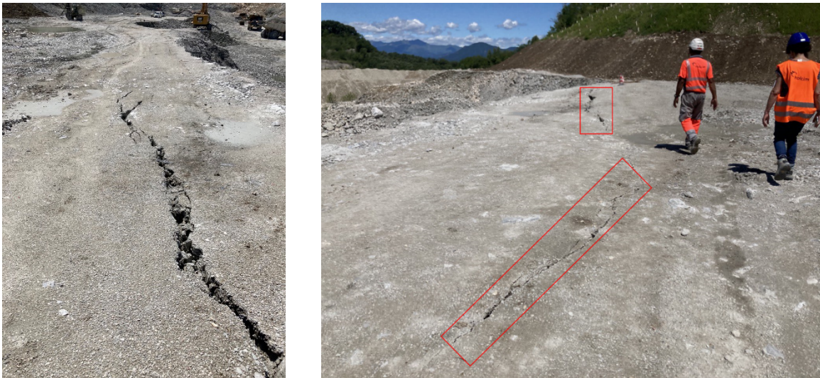
Figure 2. Example of tension cracks formed at the edge of the bench after blasting.
