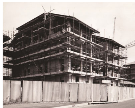
Figure 9. One of the Borini buildings under construction, ca. 1967 (photo by R. Moncalvo) (ATC, 19447).
