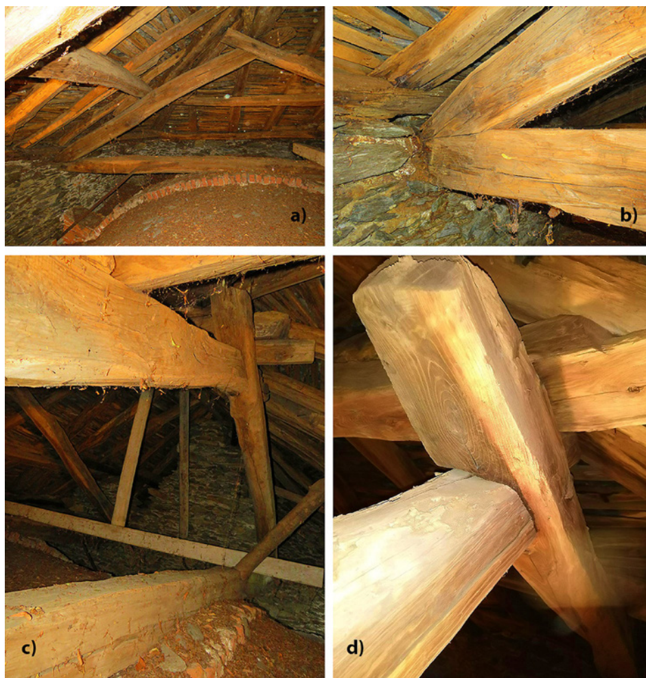
Fig. 5. (a) North truss; (b) detail of the tie beam-rafter connection, in evident degradation inside the masonry support; (c) tie beam rests on the extrados of the vaults; (d) detail of a half-lap coupling connection.
