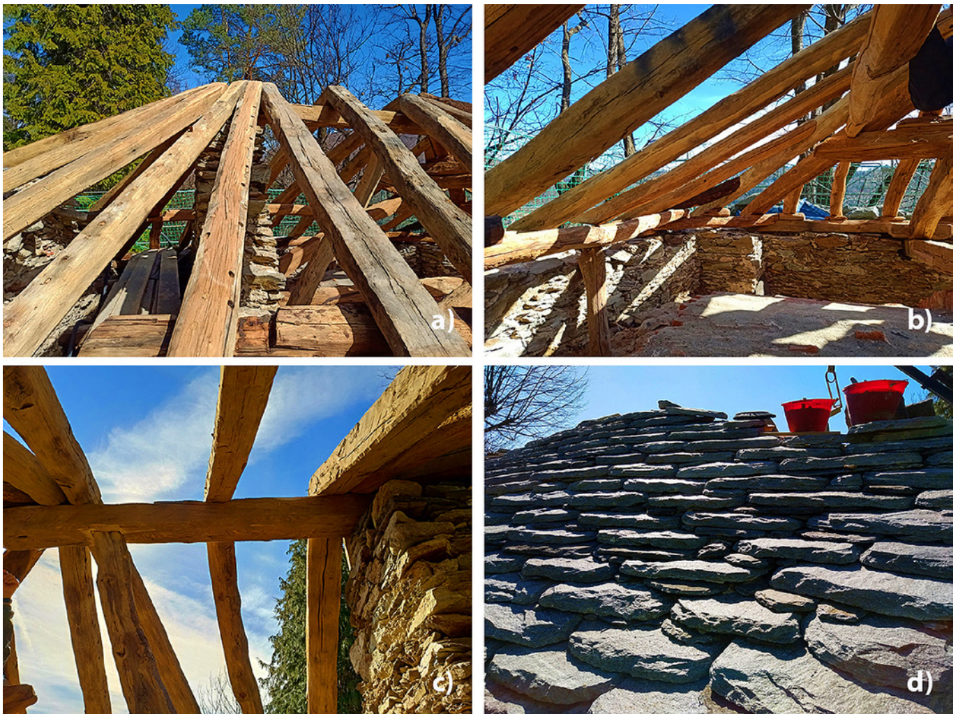
Fig. 10. (a) Placement of new timber elements alongside the original ones cleaned up; (b) integration of the new quay beams into the original structural scheme; (c) cleaning and static improvement of the area around the ridge beam; (d) reconstruction of the original stone roof covering.
