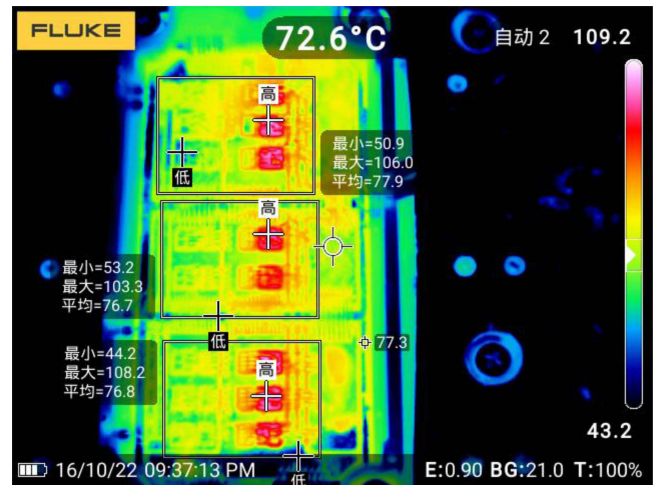
FIGURE 15. Steady state infrared temperature distribution.
