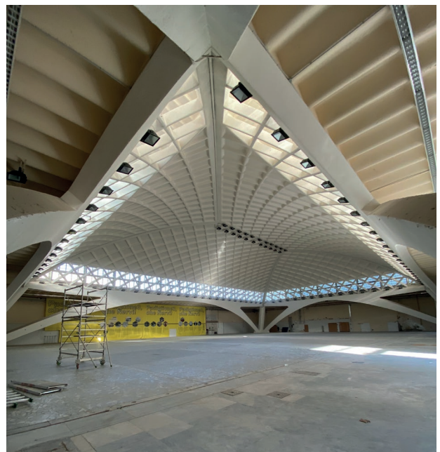
Figure 2 | View of the interior of Hall C, where it is also possible to appreciate the detail of the inclination of the arches supporting the vault and perimeter slabs.
