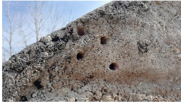
Figure 95 : Rotten hemp-lime on northern top
