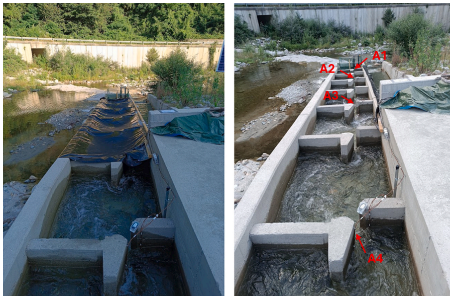
Fig. 2. The vertical slot fishway in covered (left) and open (right) conditions. In the foreground the uppermost antenna (A4) and test tag are visible on both photos. The position of the four antennas (A1–A4) is indicated in red on the right. (For interpretation of the references to colour in this figure legend, the reader is referred to the web version of this article.)
