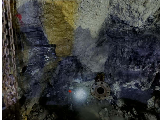
Figure 12. Roof permeable phenomenon.
