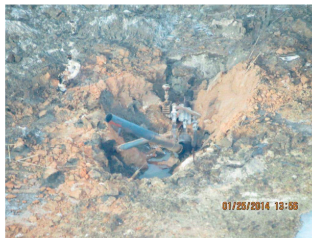
Figure 1. Uplift of the valve and pipeline section following rupture and explosion. Photo credit: courtesy of Transportation Safety Board of Canada [26].
