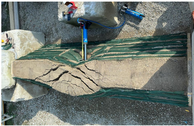
Fig. 11 Tension crack pattern developed on the top of both embankments. The photo refers to System B
