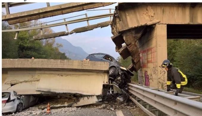
Figure 1-2: Collapse of the Annone overpass.
