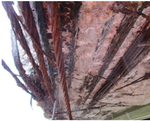
Figure 5-9: Real damage on the side beam.
