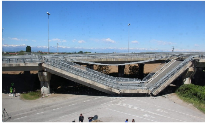
Figure 1-3: Collapse of the Fossano overpass.
