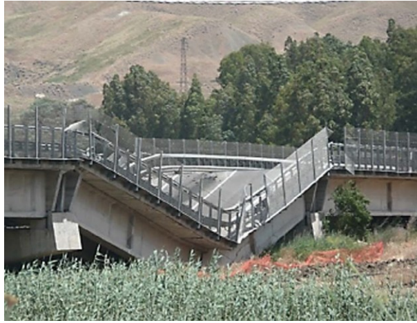
Figure 1-1: Collapse of a span of the Petrulla viaduct [3].
