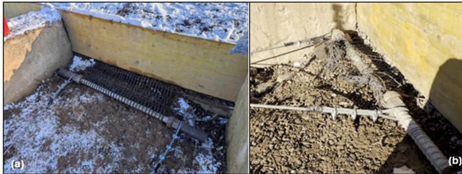
Fig. 7. Connection of the geogrid for force transmission: a) Initial method with stitching of the meshes one by one; b) Tying of the longitudinal filaments.
