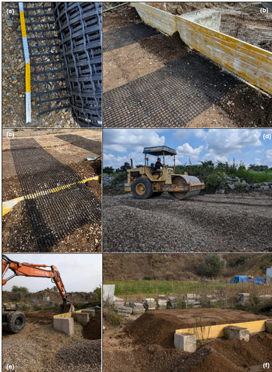
Fig. 4. Testing embankments. a) Geogrids; b) and c) Placement of geogrid strips and wooden containment forms; d) and e) Construction phases of the experimental embankments; f) View of the first completed embankment.
