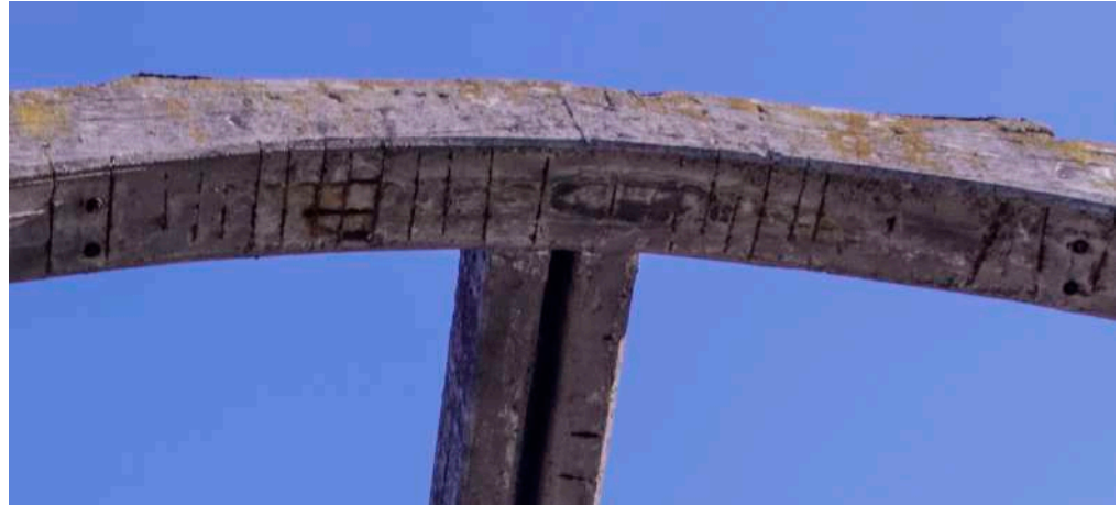
Figure 9. Example of exposed iron located in the intrados of the concrete arch.
