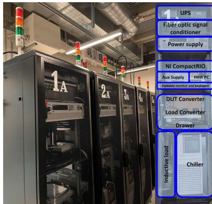
(b) Left: 6-unit, 19" industrial rack array; right: detailed configuration of one rack. Fig. 2. DC- and AC Power cycling test setup.
