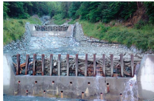
Fig. 3 The check dams in Pèriere filled after the July 11 th 2016 debris flow event.
