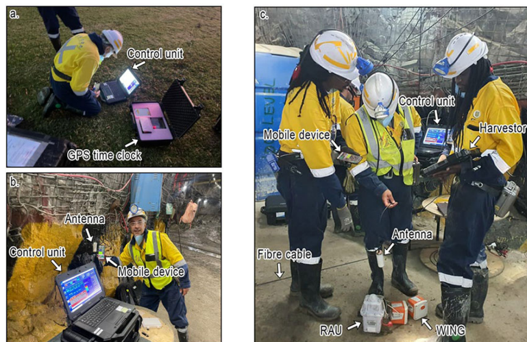
Figure 4— (a) The GPS time system is synchronised with satellites for underground tunnel use, providing signals to (b) Mobile devices at 3000 m below the surface, and (c) Fed to nodal systems
