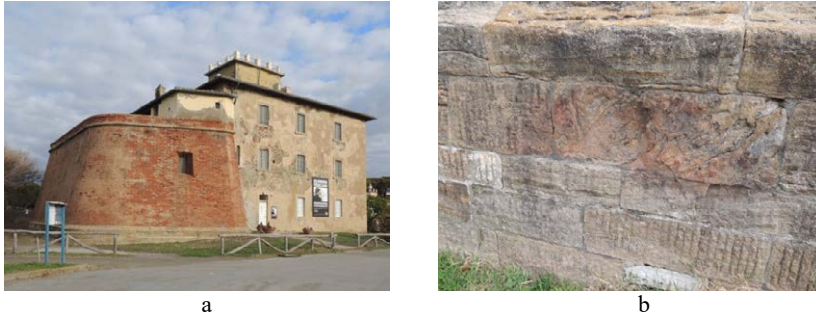
Figure 4 – Forte di Marina di Bibbona (a); particular of exfoliation phenomena caused by improperly installed Pietra Panchina (b).
