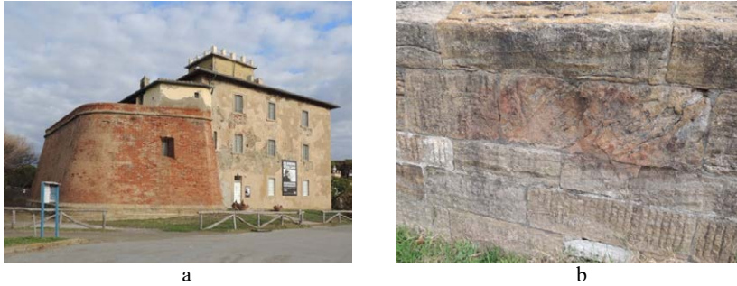
Figure 4 – Forte di Marina di Bibbona (a); particular of exfoliation phenomena caused by improperly installed Pietra Panchina (b).
