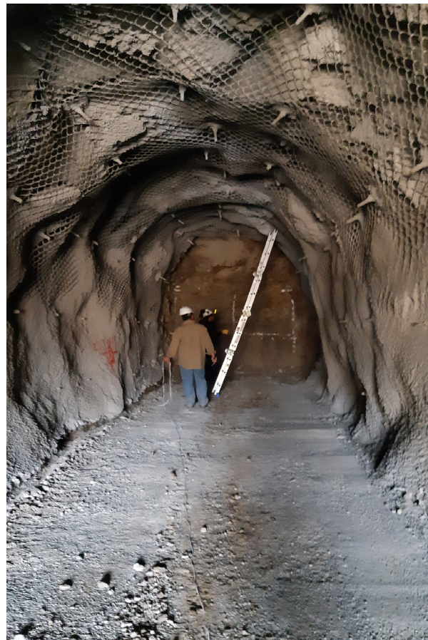
Figure 4. Inside view of the tunnel. The heads of the rock bolts are clearly visible on the vault of the tunnel.
