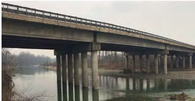
Fig. 5 Photograph of the first 3 spans of the Stura river bridge (Turin-Caselle direction)
