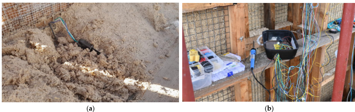
Figure 6. Pictures showing the work of placing the probes: (a) embedding the probes and (b) welding the hardware system.
