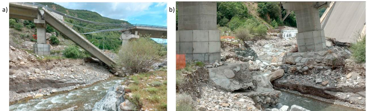
Figure 1. Collapse of the Longobucco bridge, near Cosenza: a) Collapsed deck span and rotated pier; b) Detailed view of the foundation of the rotated pier.
