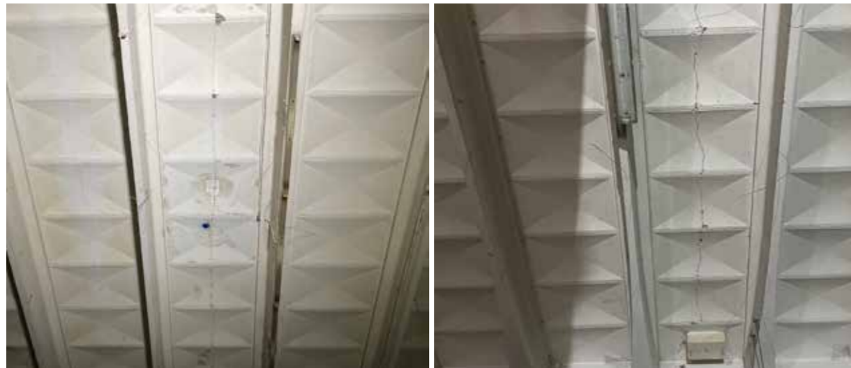
3c 2.1: Two examples of cracks running along the longitudinal direction of reinforced concrete ceiling panels. To be clearly visible even simply in a photo, the light from the flash had to pinpoint the anomaly, hence the difficulty to use photogrammetry
