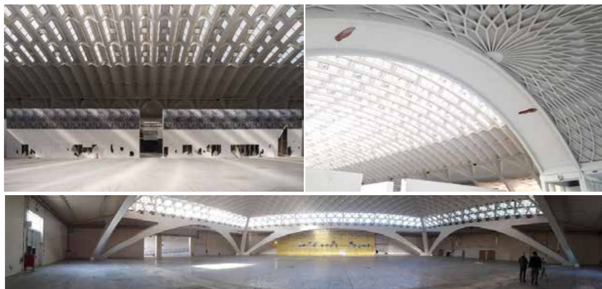
3a 3.3.a, b, c: Interior environments object of the 3D detailed survey methods using traditional laser scanning techniques, a hybrid technique from the Swift mobile system and terrestrial photogrammetry for the structural elements and related diagnosis.
