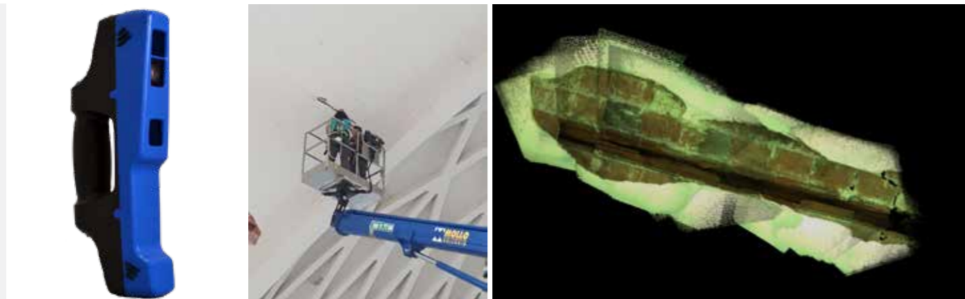
3a 9.8: Stonex F6 SR - The forklift made it possible to reach distances of less than one meter in the great arch that separates the central nave and exedra. A portion of the surface where the investigations operated on the cleaning and removal of plaster due to a pre-existing crack was acquired on a very large scale, as can be seen from the preview shown in the photo.
