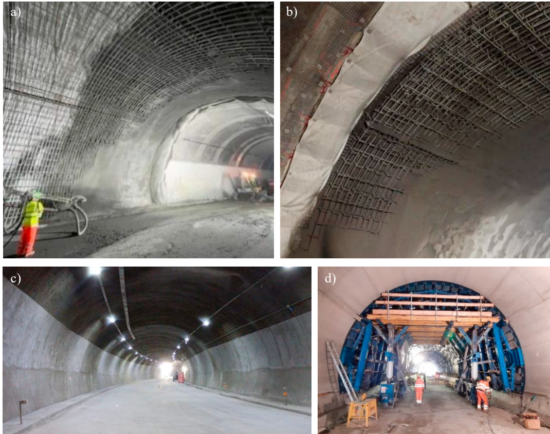
Fig. 8 a) and b) “Manfreida” tunnel construction site – relining by high strength shotcrete, c) Relining by high strength shotcrete - Pilot application at “Manfreida” tunnel, d) Relining by high strength fibre reinforced plain concrete - Pilot application at “Colle” tunnel
