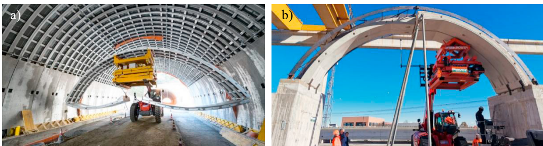
Fig. 9 a) Relining by liner plates - Pilot application at “Castello” tunnel, b) “Poderuzzo” tunnel - Field test of pre-cast concrete shell implementation
