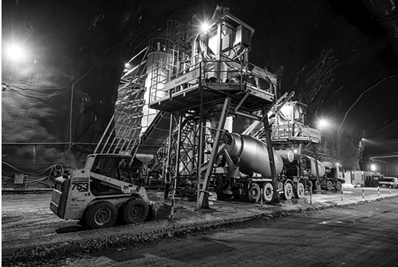
Figure 6.21 Underground batching plant located in a logistic cavern. (Courtesy of BBT-SE.)
