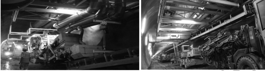
Figure 6.18 Telescopic ventilation platform for fresh air supply, allowing efficient suction ventilation of blasting fumes as well as increased working safety, thanks to free floor space for working and parking.
