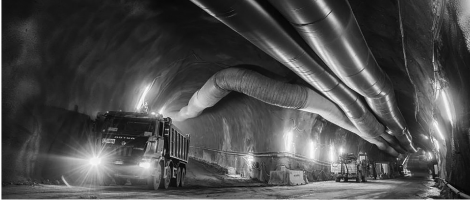
Figure 6.56 Ventilation ducts in the Mules adit.
