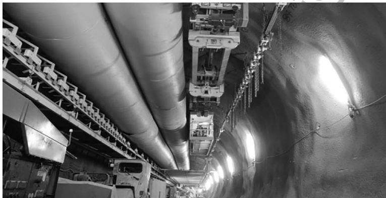
Figure 6.19 Monorail for direct supply of the heading area.
