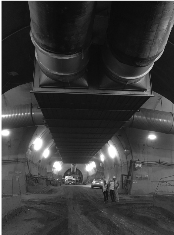
Figure 6.58 Ventilation plenum installed in logistic chamber (adit end).
