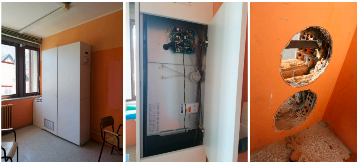
Fig. 1. (a) one of the installed DMV units; (b) the system controlling board; (c) a moment of the installation.
