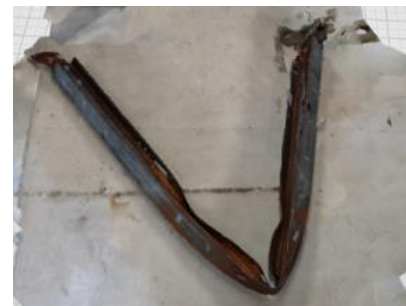
Figure 1(b). Deformed steel post
