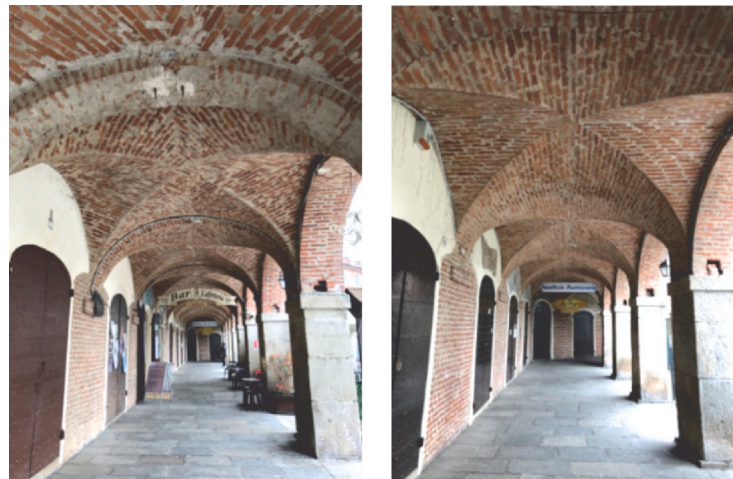
Fig. 2. View of two different 18th century vaults of the portico, with radial masonry pattern (right) and diagonal pattern (left).
