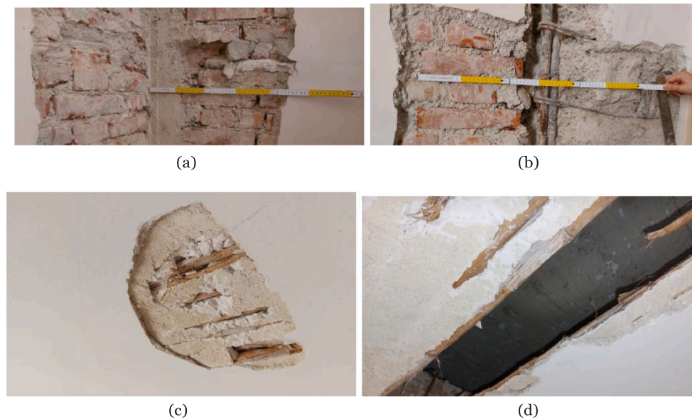
Fig. 4. (a) View of the CM structure and (b) a typical vertical RC element. (c)–(d) show the intrados floor.
