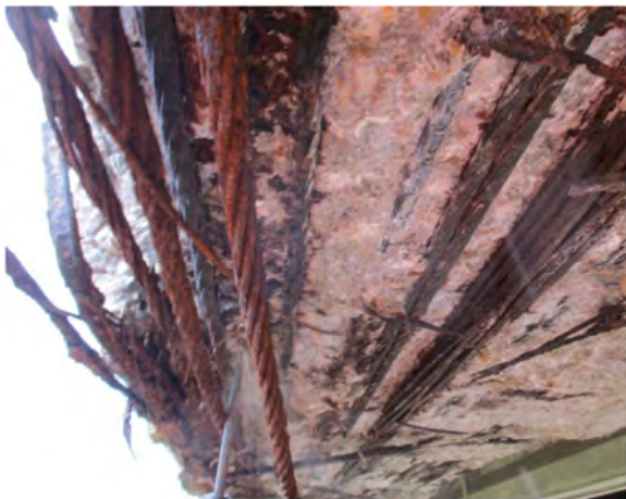
Fig. 10. Real damage on the side beam.
