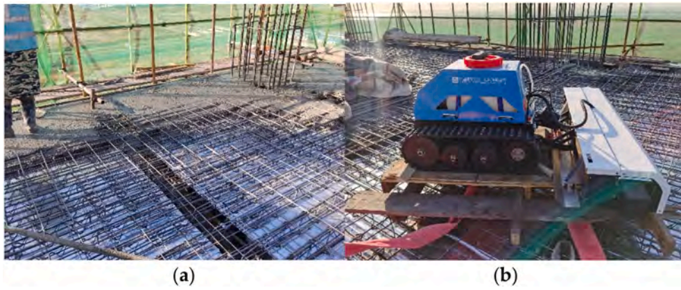
Fig. 14. Field test of concrete curing robot: (a) Engineering appearance of concrete curing site; (b) Concrete curing robot body.
