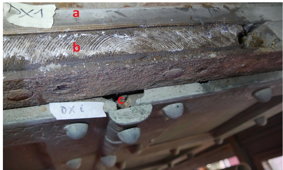
Fig 5. The upper side of the right leaf of the San Clemente door. a) The first layer of horizontal planks. b) The second layer of planks placed vertically: the annual rings on the cross section are highlighted with chalk powder. c) The gap through which a third layer of wood could be glimpsed.
